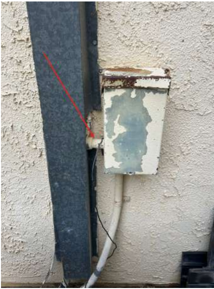
Photo 5.1C - Cooling system — operated via normal controls
