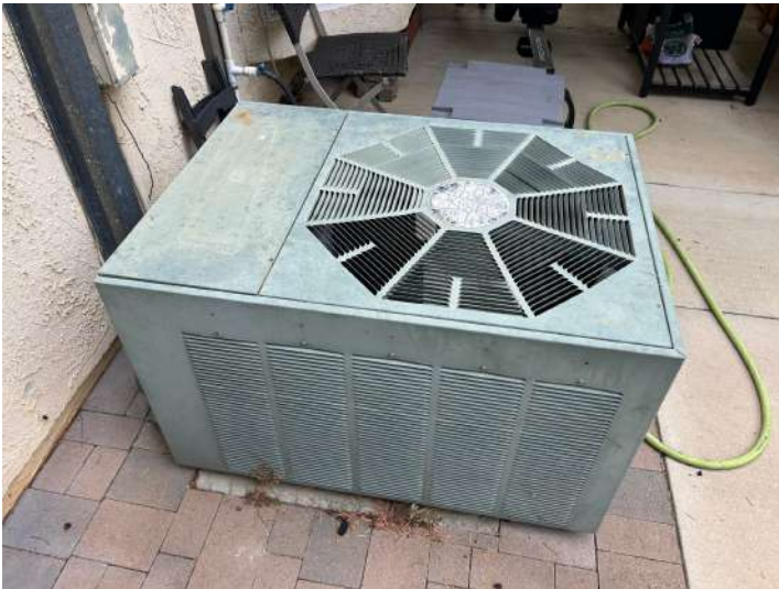
Photo 5.1A - Cooling system — operated via normal controls
