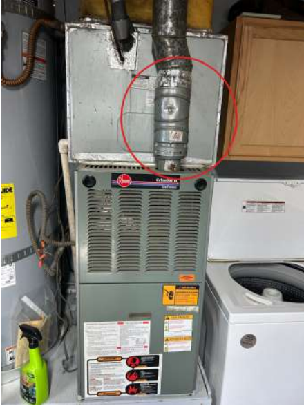
Photo 4.1A - Heating system — operated via normal controls
