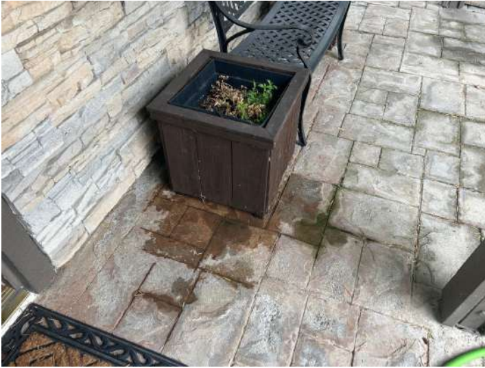
Photo 3.6A - Active water penetration
