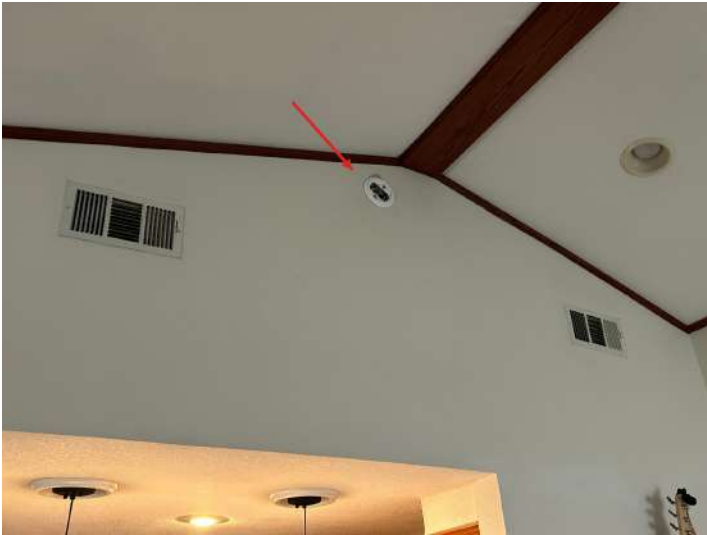
Photo 7.10A - Smoke & CO detectors — presence verified
