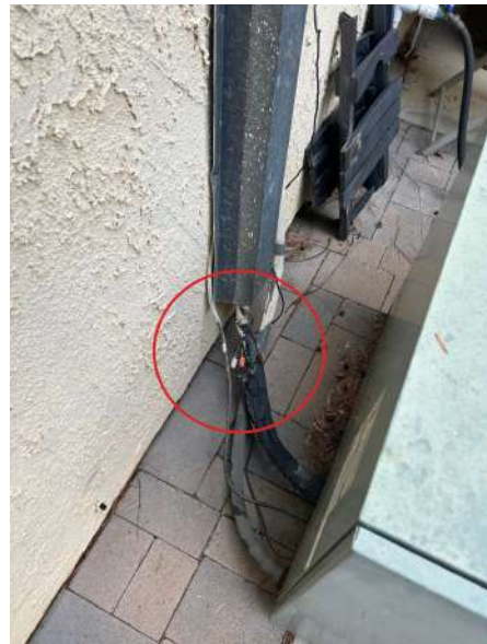
Photo 5.1B - Cooling system — operated via normal controls
