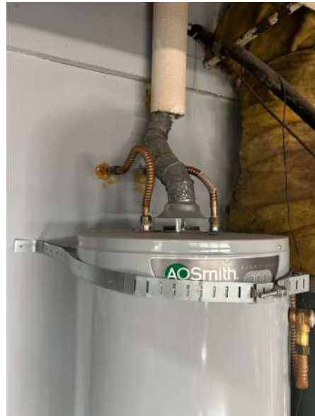
Photo 6.3B - Water heater — energy source, venting, TPR valve, seismic bracing
